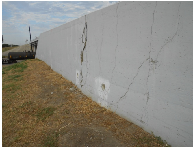
Figure 2.8 Failure of a low wall over highway loop 12, in Dallas, Texas due to sliding movement
